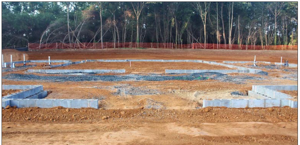
Clockwise from upper left: Earth is moved in preparation for construction (Photo: Bob Martin); builder Helen Cantrell shows plans to Carl Little and Mike Logan; a group of UUFFers stands in the gathering space between the front door and the Fellowship hall; the arrow on this aerial view points out our location, with Pratt Park to the right, the YMCA below, Chatham above, and Chatham Heights Road to the left; footers and block in place show outline of building looking in from the front door (Photos: Suzanne Logan).
